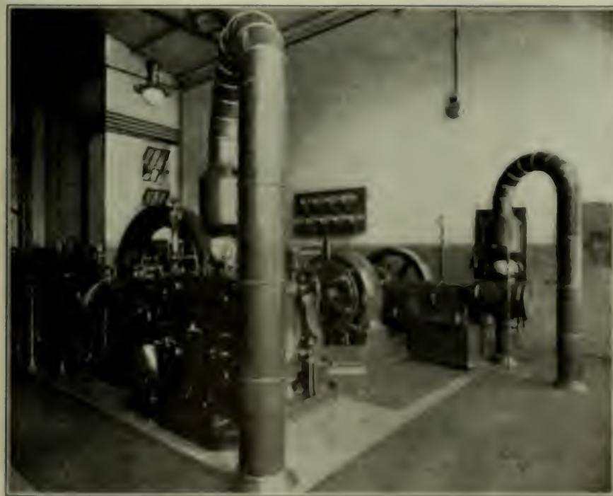
16X30 MURRAY-CORLISS AND 125172 BRK CITY IRON WORKS ENGINE, WITH 250 AND 70-KILOWATT SHELL GENERATORS
